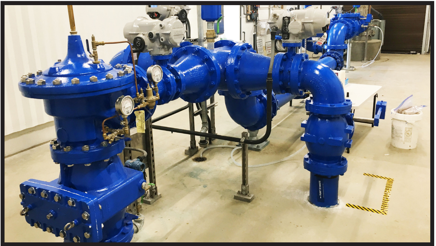
2019 ACEC California's EEA Golden State Winner: Woodland Aquifer Storage and Recovery Wells #29 and #30 (Carollo Engineers, Inc.)
