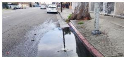
Curb & Gutter in need of repair
