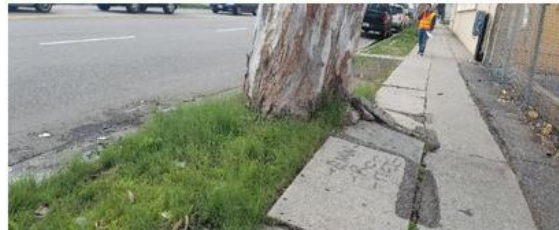
Sidewalk in need of repair / Tree Replacement
